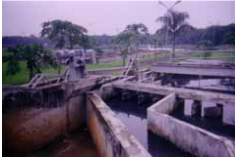
Gambar III. 8. instalasi IPAL "Pemisah pasir"
