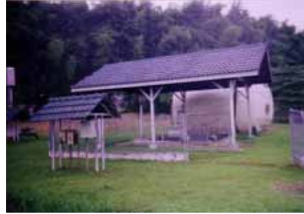
Gambar III. 9. instalasi IPAL UASB (Upflow Anaerobic Sludge Blanket)
